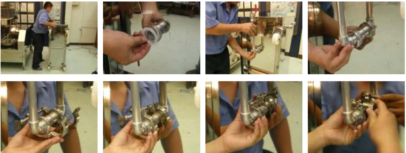
水槽排水管連接 The combination of the water trough drain pipe.
