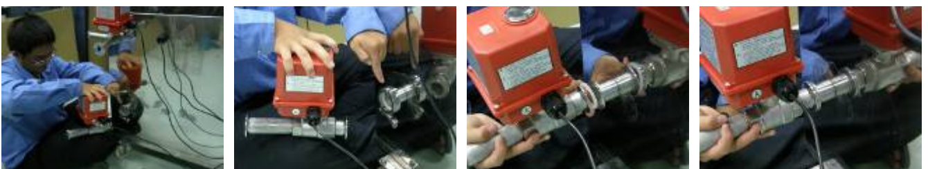
(4) 排水二通閥與水槽連接 The installation of auto two way valve installation (drain water)
